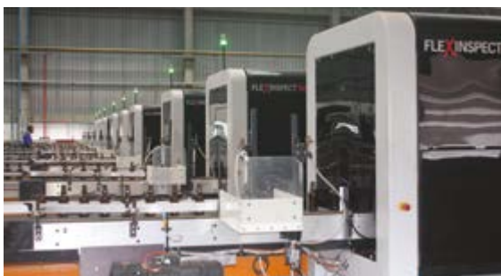
Nine FlexInspect T and nine FlexInspect BC machines were installed during the third quarter of 2014.
